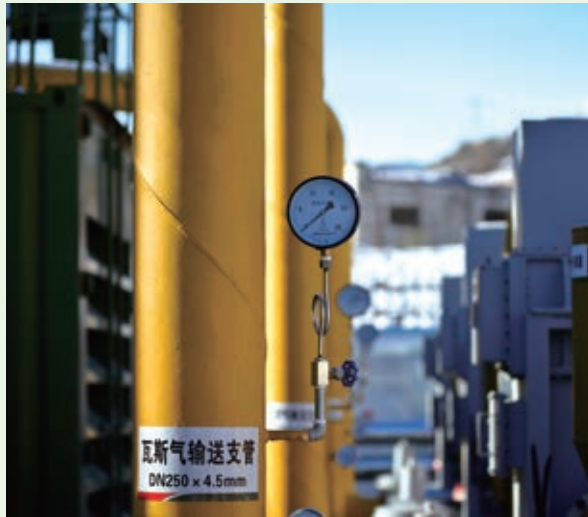
Methane power generation project of Liuhuanggou Coal Mine
