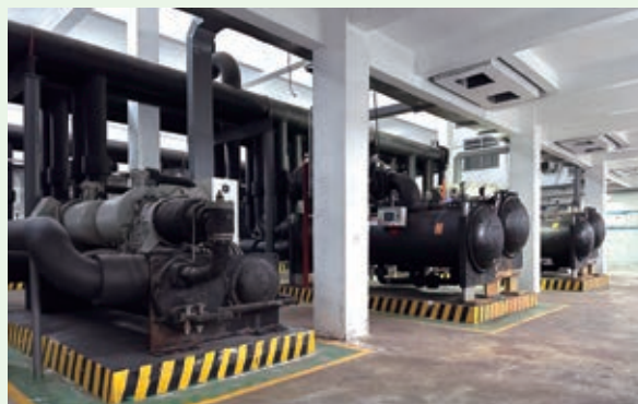
The comprehensive mine waste heat utilisation project of Lilou Coal Mine
